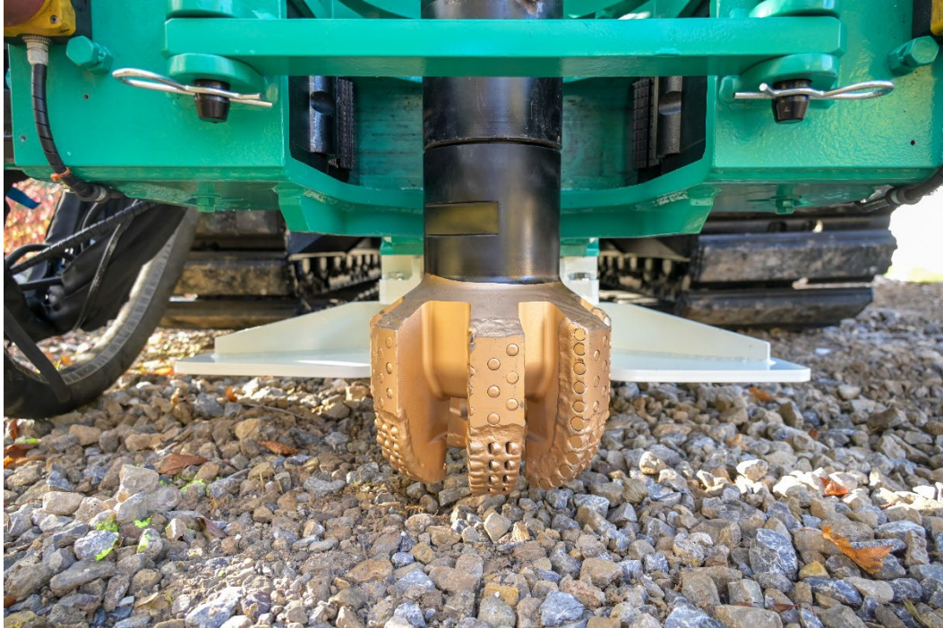
Figure 7: F-IEG drilling rig Hütte HBR 207 GT showing a 12 ¼ “-PCD bit attached to heavy drill collars in order to realize a preferably vertical pathway without using any additional (cost-intensive) Rotary Steerable System tools
