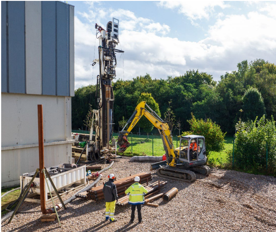
Figure 6: Drilling setup at the demo site showing the drilling fluid circulating system
